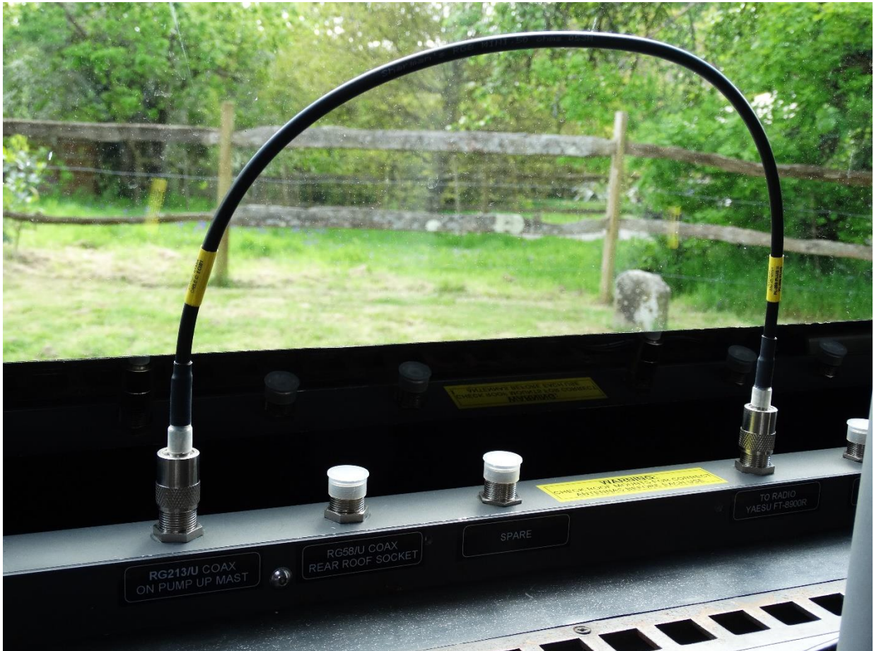
Don't take all of your antenna cables directly to the back of the radios, instead use a patch panel which will allow the easy and quick installation of new radios and the patching to new antennas from existing radio equipment. Keep connectors common (here we see all PL259 being used) and label everything.
